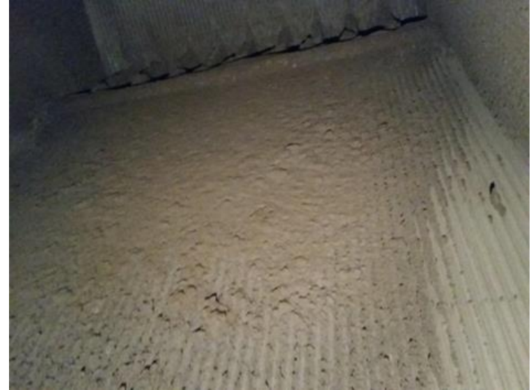
Rear wall of the 2 nd duct against the flow direction in the direction of the 1 st duct photographed
